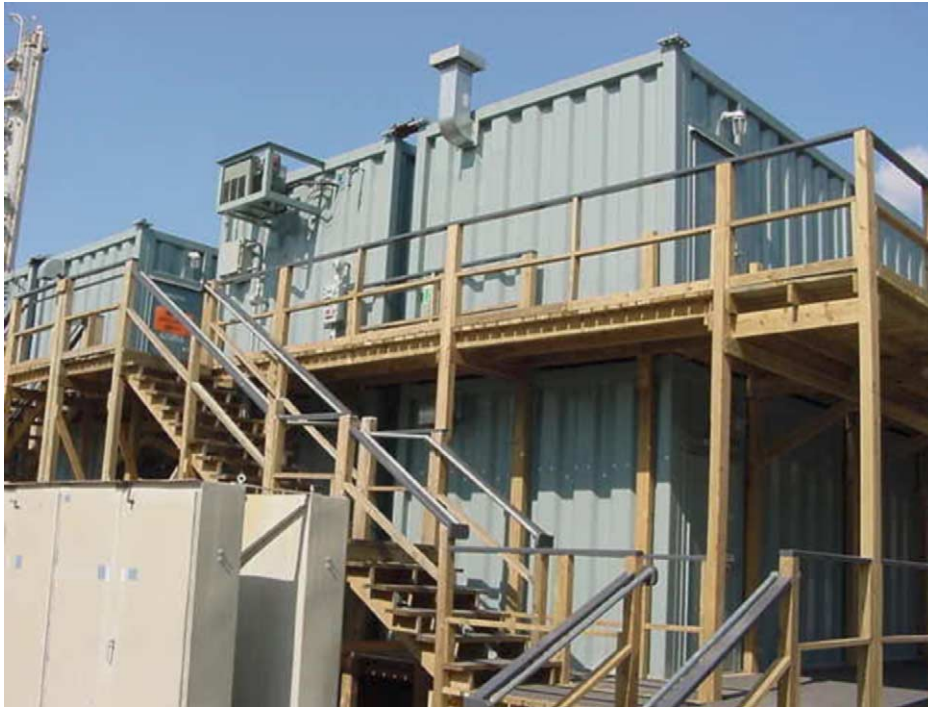
Fig. 6. Stacked complex of BRPBs.
